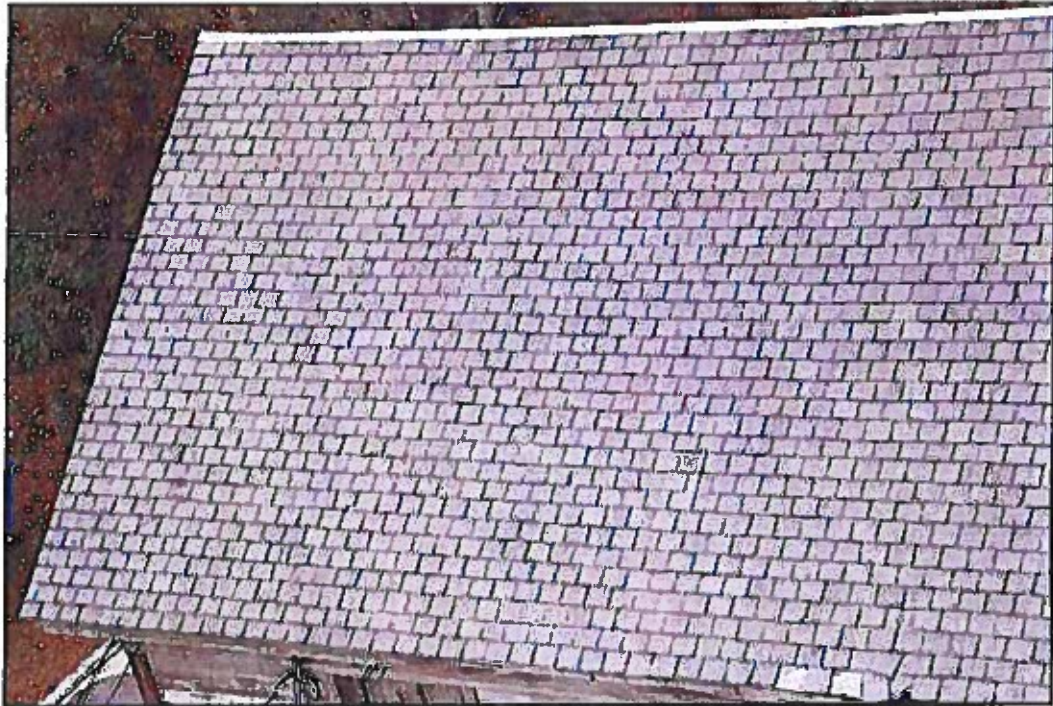
Photo 3: South pitch of ell barn roof. Note missing slates at lower right have caused considerable rot in the cornice directly below.
