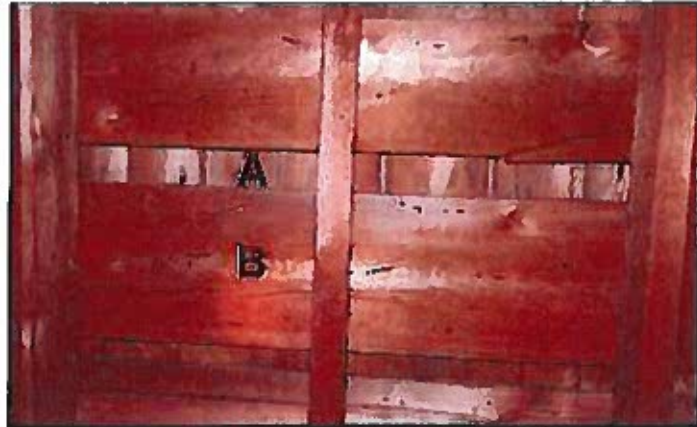
Photo 7: Underside of roof from left showing original wood shingles (A) installed on the original spaced roof boards (D). Nails visible on underside of boarding are from shingles. Slate nailing is primarily held by wood shingles.
