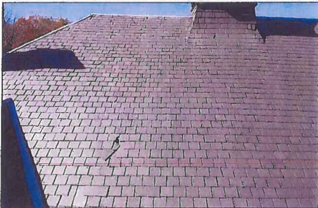
Photo 2: Southern end of east roof pitch. Only a few shingles show defects.
