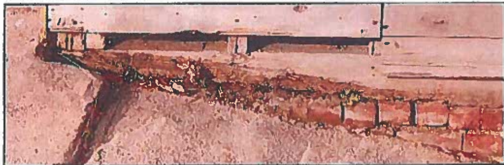
Photo 37: Sill at south facade of main barn to right of door. The face of the sill has rotted. Its condition and treatment need further investigation, similar to the sill in photo 35.
