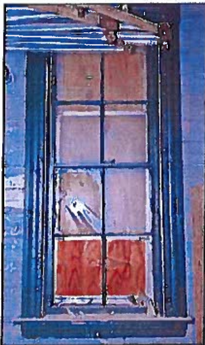
Photo 49: Interior side of first floor main barn window showing molded casings that should be retained and preserved. Sash are intact and can probably be retained with new glass and glazing.
