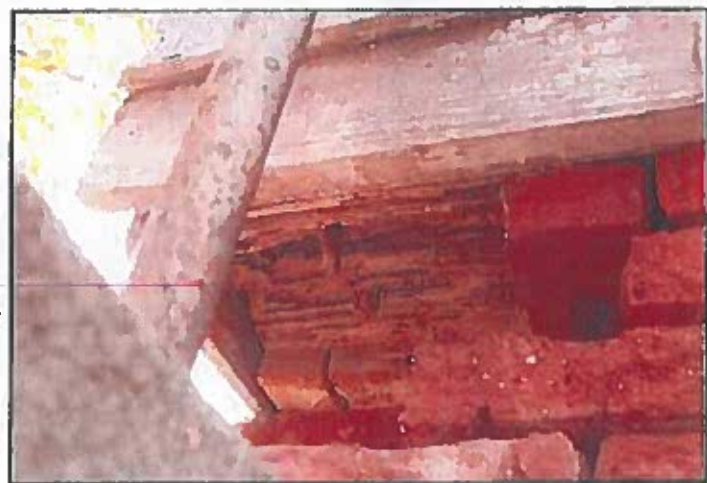
Photo 38: Sill at southeast corner of main barn. The underside of the east sill has lost several inches from insect damage and rot, while the south sill remains sound. The core of the east sill above the damage seems to be sound, and the visible damage only extends a couple of feet to the right. However, further probing should be done to verify the extent of damage. The sill needs to be repaired by piecing in sound wood to replace the deteriorated material, and the brick foundation rebuilt down to sound brick and mortar. In this case the full 12" depth of the wall need rebuilding at the top.
