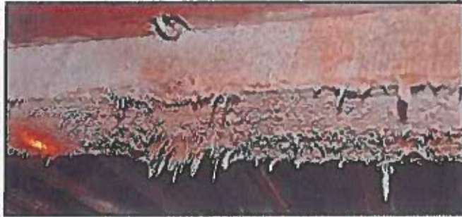
Photo 77: Main ceiling beam in basement of main barn showing area of fungal decay that is probably "white rot" as opposed to the more dangerous "brown rot".
