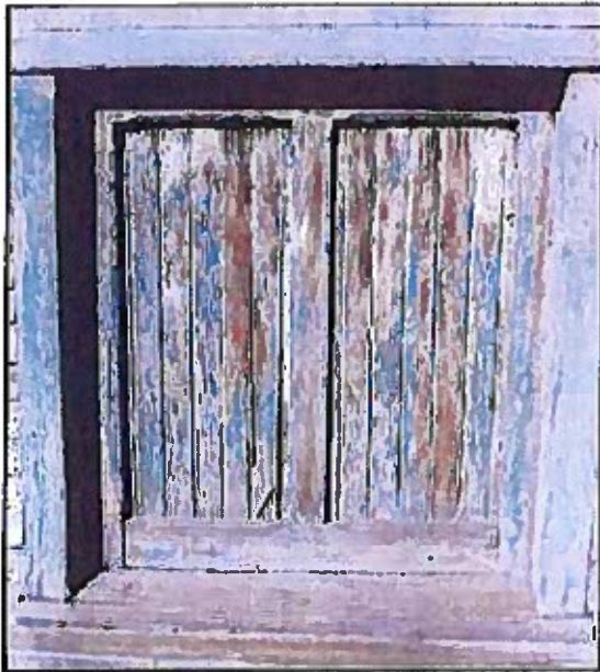
Photo 47: Original loft door of ell barn south facade. There are two original doors which should be retained and preserved. They are functional but have weathered surfaces and will need some carpentry repairs.
