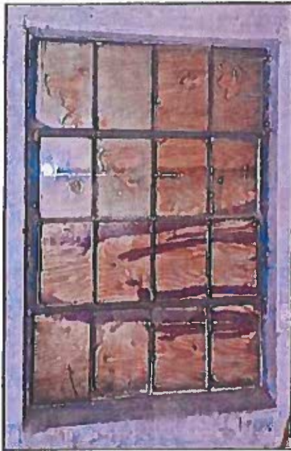
Photo 51: Interior side of old basement steel window with substantial rust. Replacement with new wood or metal window matching the size and pane configuration would be acceptable.
