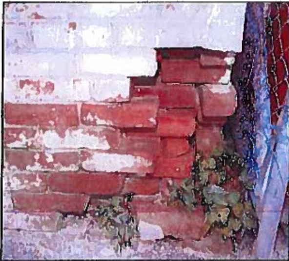
Photo 58: Foundation at northeast corner of main barn with loose and missing brick. This section should be rebuilt with matching brick.
