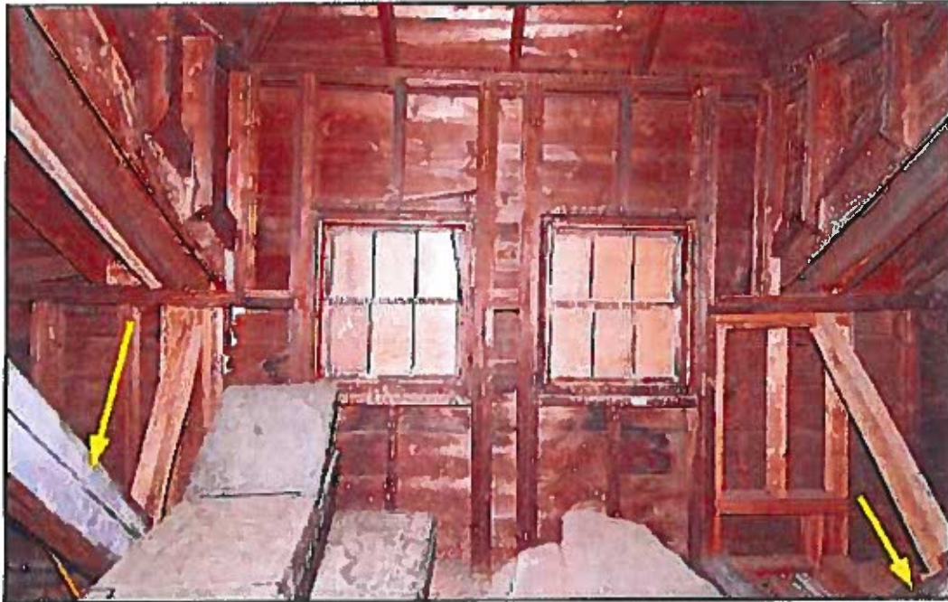
Photo 73: Interior of dormer #4 at east wall of main barn showing past repairs to stabilize framing rotted by former roof leaks. The ends of the upper truss rafter chords (arrows) appear to be rotted completely off where they were originally joined to the floor beams forming bottom truss chords.
