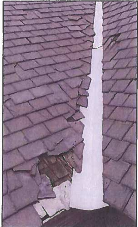
Photo 12: Slate defects - Substantial number of broken slate at south valley between ell barn and main barn roofs risks major water damage to framing below roof and should be repaired as soon as possible. Aluminum valley remains intact. Note wood shingles under missing slates.
