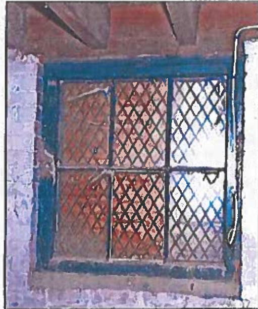
Photo 52: Interior side of main barn basement window with intact sash and old protective grill on the exterior. Both the sash and the grills should be retained when the sash is intact.
