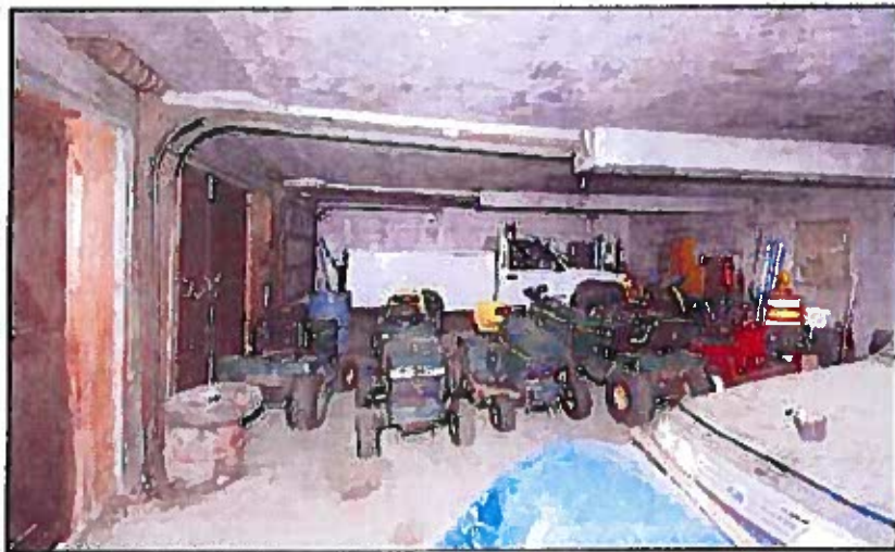
Photo 67: Interior of ell barn first floor showing cement plaster wall and ceiling finishes. Heavy vehicles such as the truck at the end wall should not be stored on this floor until its condition has been evaluated by a structural engineer (see Photo 63)
