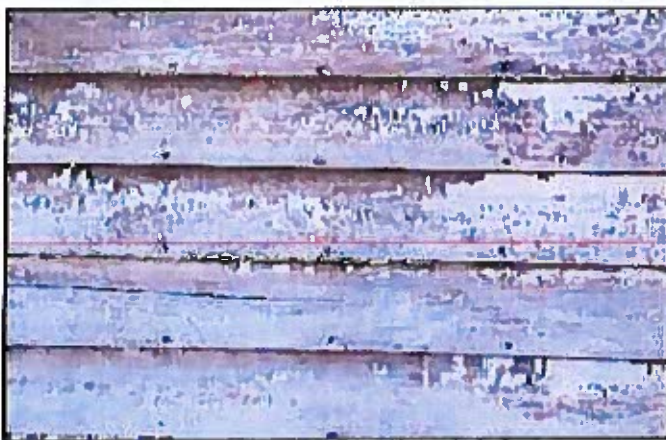
Photo 34: Typical clapboard conditions at north facade of main barn; weathering is moderate and splits are less severe and less frequent. Retaining the existing clapboards in place is feasible with replacement limited to badly split ones and the areas of missing clapboards around the windows.
