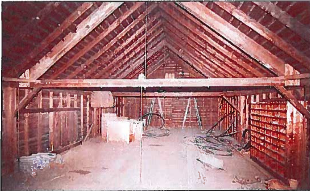
Photo 66: Interior of ell barn loft floor showing roof trusses and exposed framing. There is considerable dust and fiber debris on the floor (especially at the side walls) that is a potential fire hazard and should be vacuumed out.
