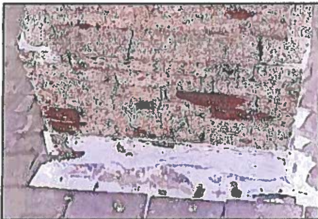
Photo 61: Chimney flashing at roof has numerous large holes that are causing leaks in the roof below.
