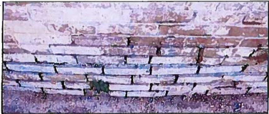
Photo 57: Brick below basement window sill of main barn east facade with open mortar joints and a number of bricks that are loose and bulging out from the wall. All the loose bricks should be taken out and reset in new mortar, and all joints in the area 100% cut and repointed using a mortar matching the relatively low strength of the existing original mortar.
