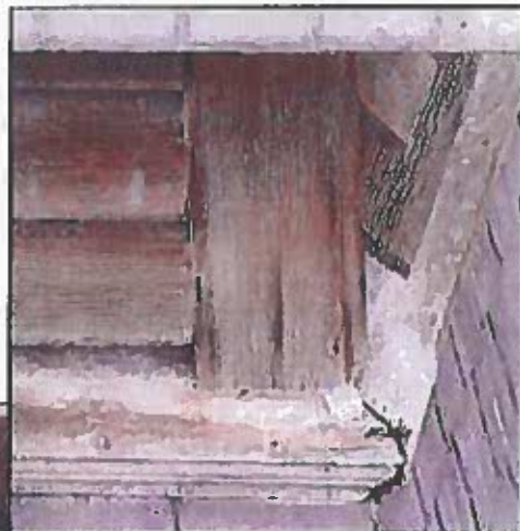
Photo 19: Detail of cupola showing gap at sill corner that was original covered with flashing, and moderate weather checking in louvers. Reflash sill corner joints. Replacement of louvers is an option, but not critical as they seem to be solid despite the weathering.
