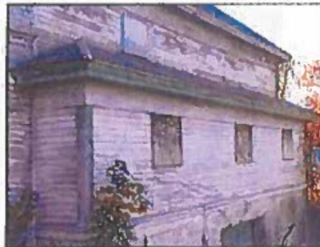
Photo 70: Overview of north ell facade showing the c. 1930s extension of the first floor. The extension does not exhibit sag of the loft wall above. However, as a precaution, the condition of sagging of the loft wall should be evaluated by a structural engineer when the basement ceiling is evaluated.
