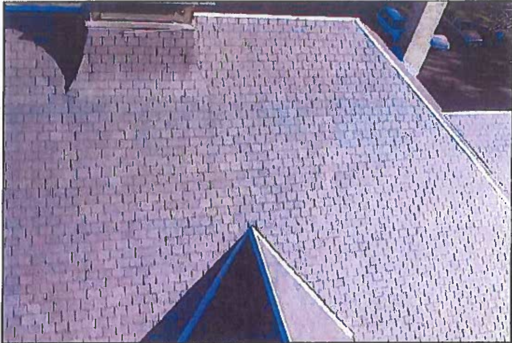
Photo 5: Southern end of west roof pitch on main barn. Only a few shingles show defects.
