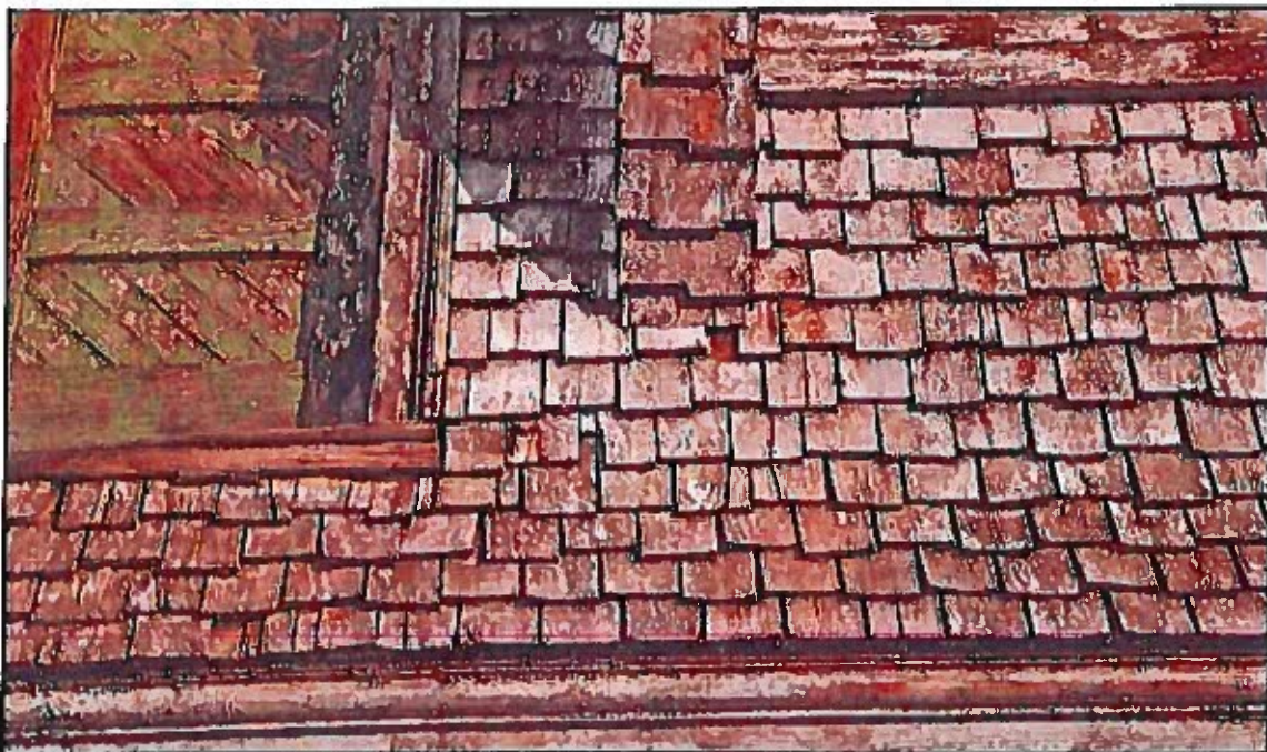
Photo 29: Shingle band adjacent to Dormer #1 on west facade showing many warped, split and missing shingles in lower portions. The extent of damaged shingles warrants complete replacement of shingles in this area, and possibly across the entire west facade.
