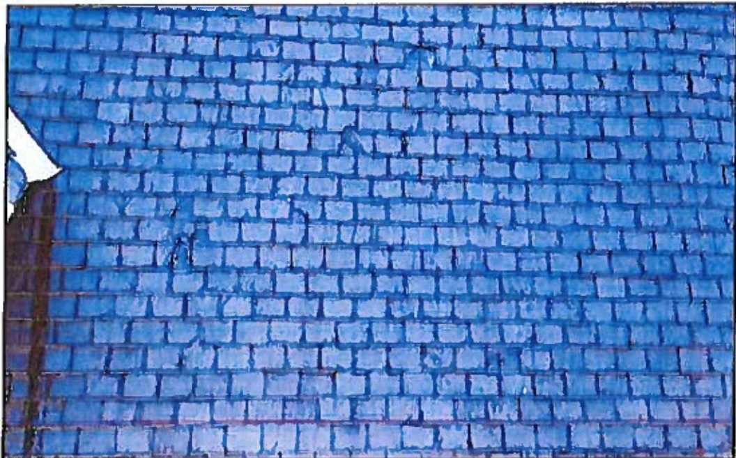
Photo 4: North pitch of main barn roof next to dormer.. This section has substantially more broken and cracked slate than other portions of the roof.
