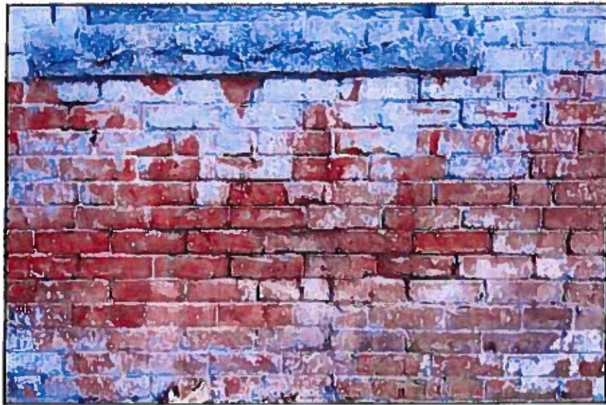
Photo 56: Brick below basement window sill of main barn east facade with open mortar joints and a number of deeply spalled (i.e., eroded) bricks. The spalled bricks should be replaced with matching new or sound salvage bricks, and all joints in the area 100% cut and repointed using a mortar matching the relatively low strength of the existing original mortar.
