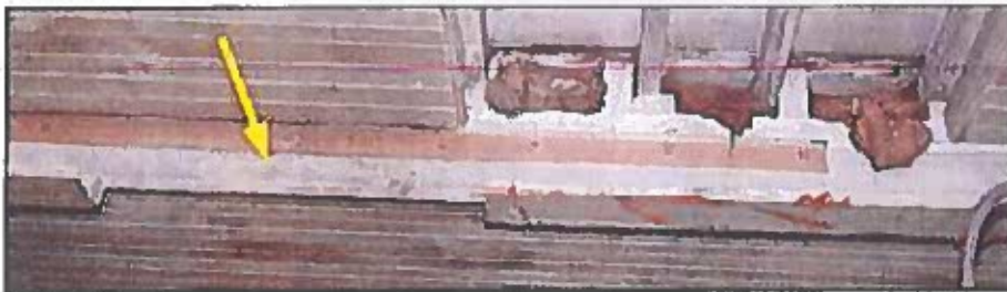
Photo 80: Bolted chord of roof trusses with section cut out (arrow). The impact of this cut on the loading capacity of the loft floor should be evaluated by a structural engineer.
