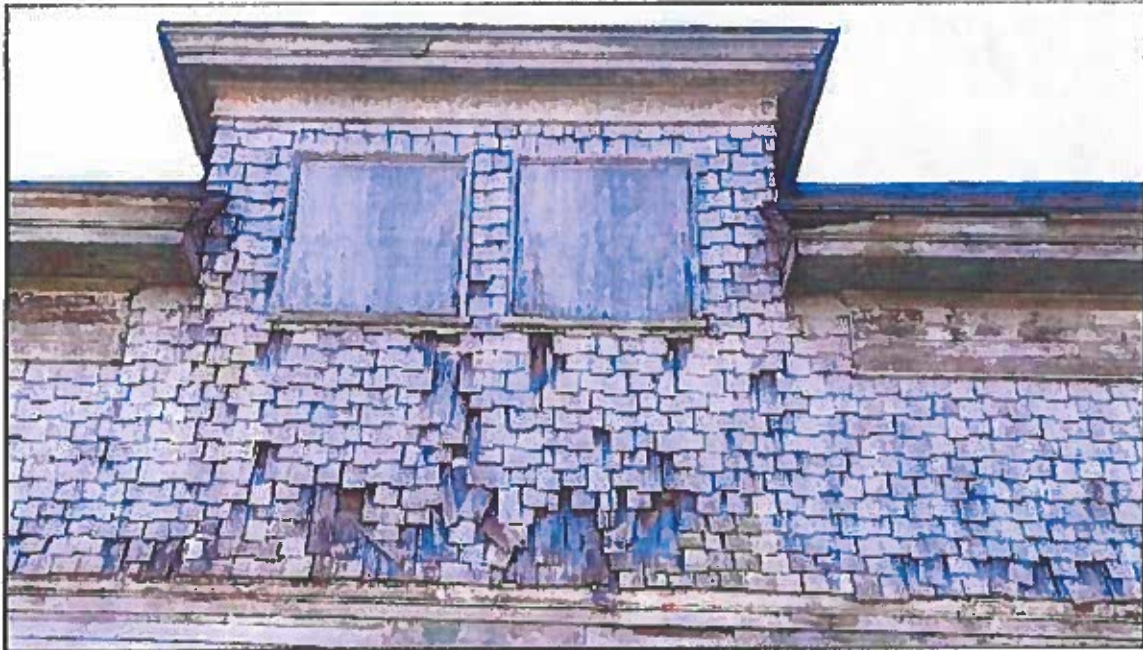
Photo 30: Shingle band adjacent to Dormer #5 on north facade showing many loose and missing shingles in lower portions. The extent of damaged shingles warrants complete replacement of shingles on this facade. Replacing only the damaged courses is not recommended as the top course of replacement shingles will not have proper cover over their nailing.
