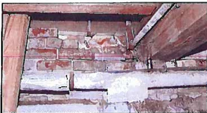
Photo 68: Basement of main barn showing obsolete steam pipes with deteriorating insulation that may contain hazardous materials. The insulation should be evaluated by a professional hazardous materials consultant and remediated as directed by the consultant.
