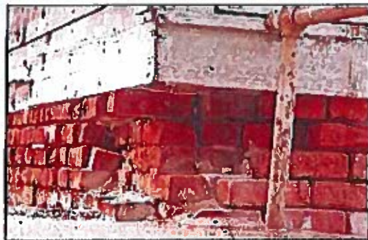
Photo 59: Foundation at southeast corner of main barn with loose and missing brick extending through the full depth of the 12" thick wall. This section should be rebuilt for the full depth of the wall with matching brick after the sill above it has been repaired.
