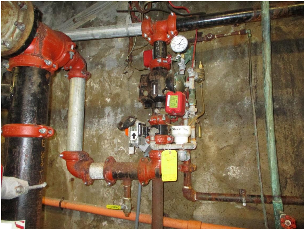
View of Wet Sprinkler System
