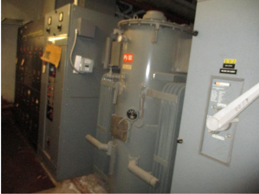
View of Electrical System
