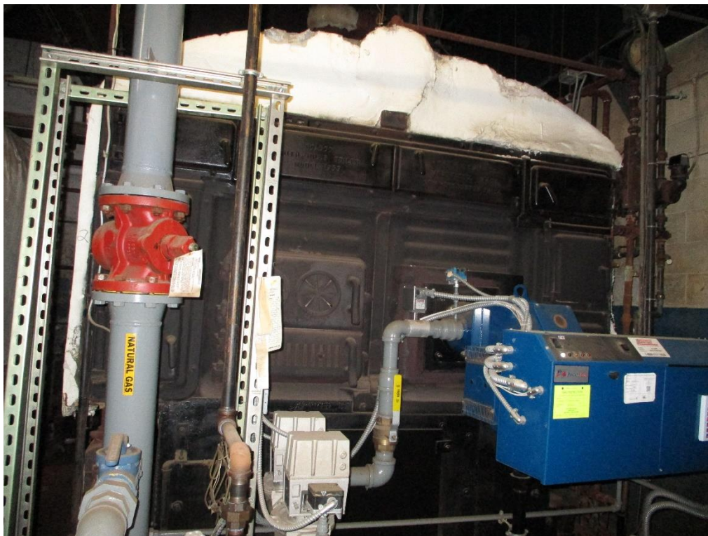
View of Boiler
