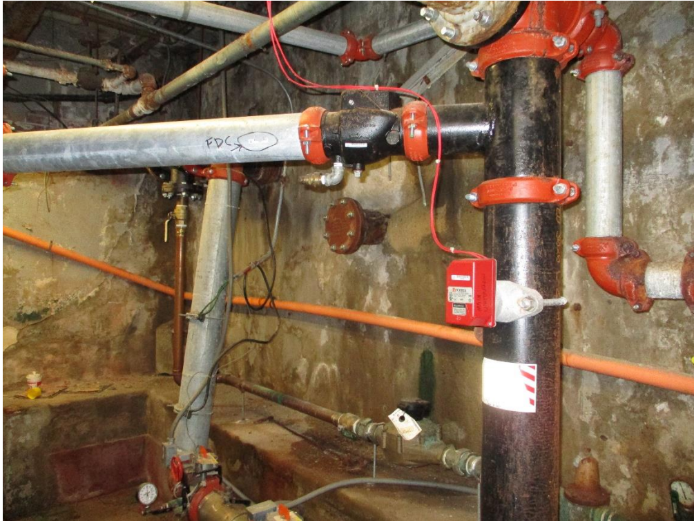
View of Dry Sprinkler System
