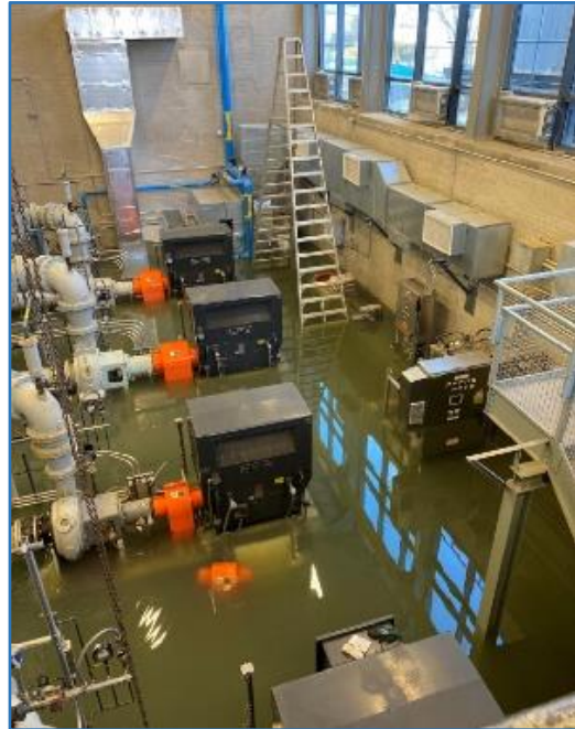
Figure 20 – A pump failure at the Lake Ave Sewer Pump station in February flooded the station and released 5.75 million gallons of untreated wastewater into Lake Quinsigamond.
